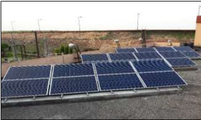
Solar PV Plant in Ash Pond.
