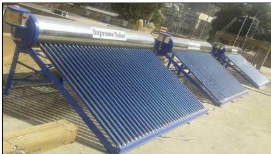
Solar Water Heater at Plant
