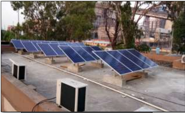
Solar PV Plant in Canteen.
